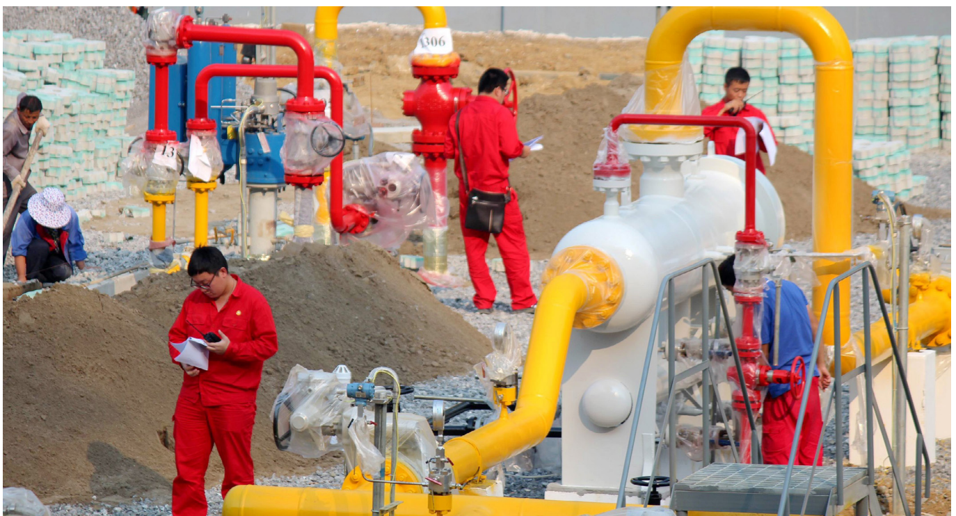
Operators test devices of the Myanmar-China natural gas pipeline in Laibin city, south China's Guangxi Zhuang Autonomous Region, 3 October 2013. The Myanmar-China natural gas pipeline was completed on 20 October 2013, further diversifying China's sources of fuel from abroad and ensuring its energy security. © Imaginechina/Corbis
